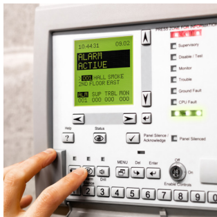
Fire facility and burglar alarm panels
